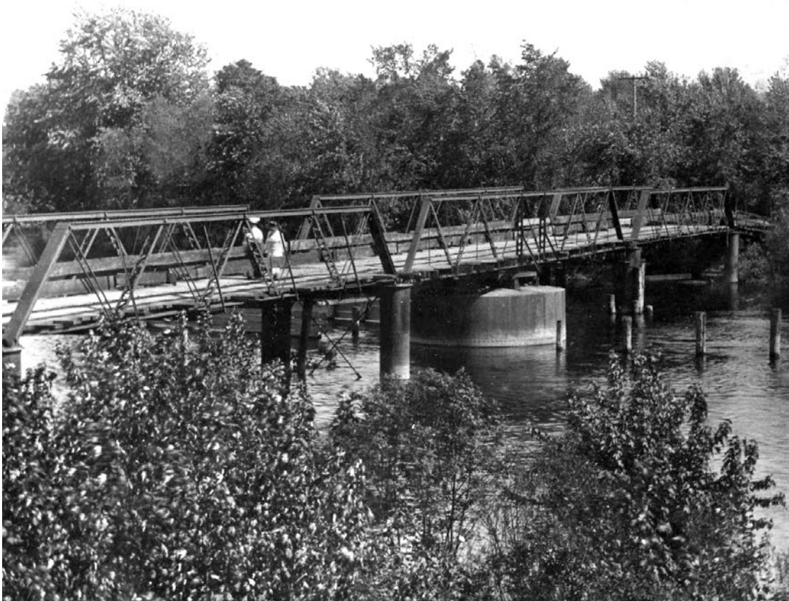
This earliest photo found in the Historical Society archives shows the New Richmond Swing Bridge as it appeared in 1915, looking much the same as it does today.
